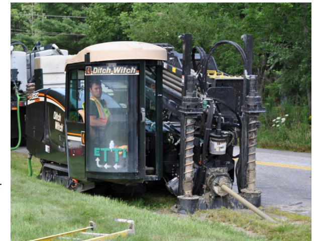
Ryan Dionne running one of ETTI's drill rigs during the Freeport/Pownal Natural Gas Project.
